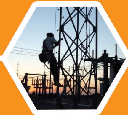
MICROWAVE/CELL SITE INSTALLATION & MAINTENANCE
